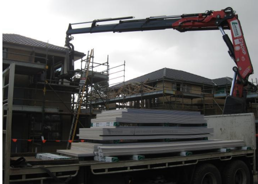
Caption: A telehandler or vehicle mounted crane eliminates the need to manually handle the plasterboard off the truck.
